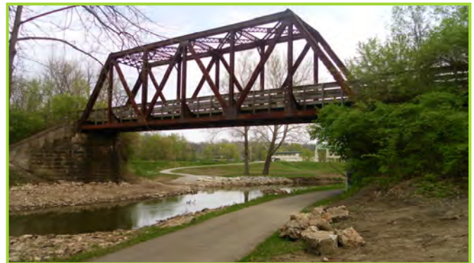
Simon Kenton Trail bridge over the Buck Creek and Buck Creek Trail (photo courtesy of Louis Agresta)
