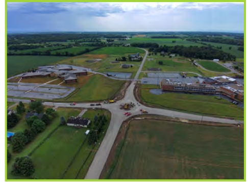
Aerial shot from the construction of the roundabout at Selma Pike and Possum Rd. (photo courtesy of the Clark County Engineer's Office)
